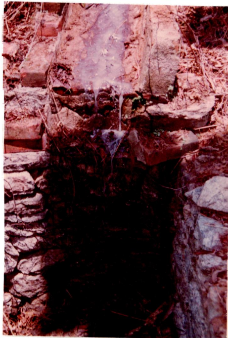
Unsightly appearance of stagnating effluent water
