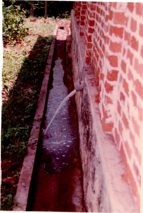
Effluent water coming out from the processing unit
