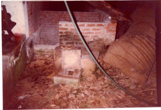
Underground plant with outside inlet and gas pipe
