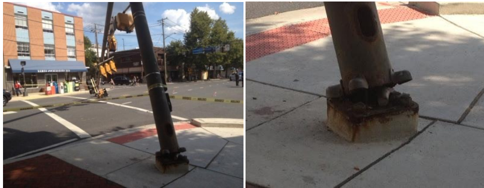
Figure 1.5 Light poles affected by corrosion
