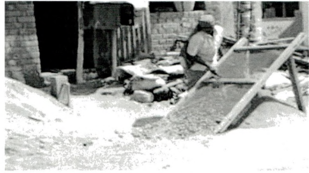
Figure 9: No Protective device before intervention
