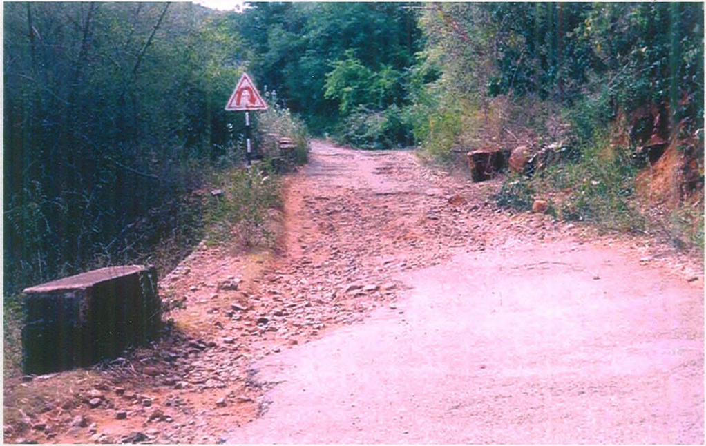
PLATE 1 ROADS IN DEPLORABLE CONDITION
